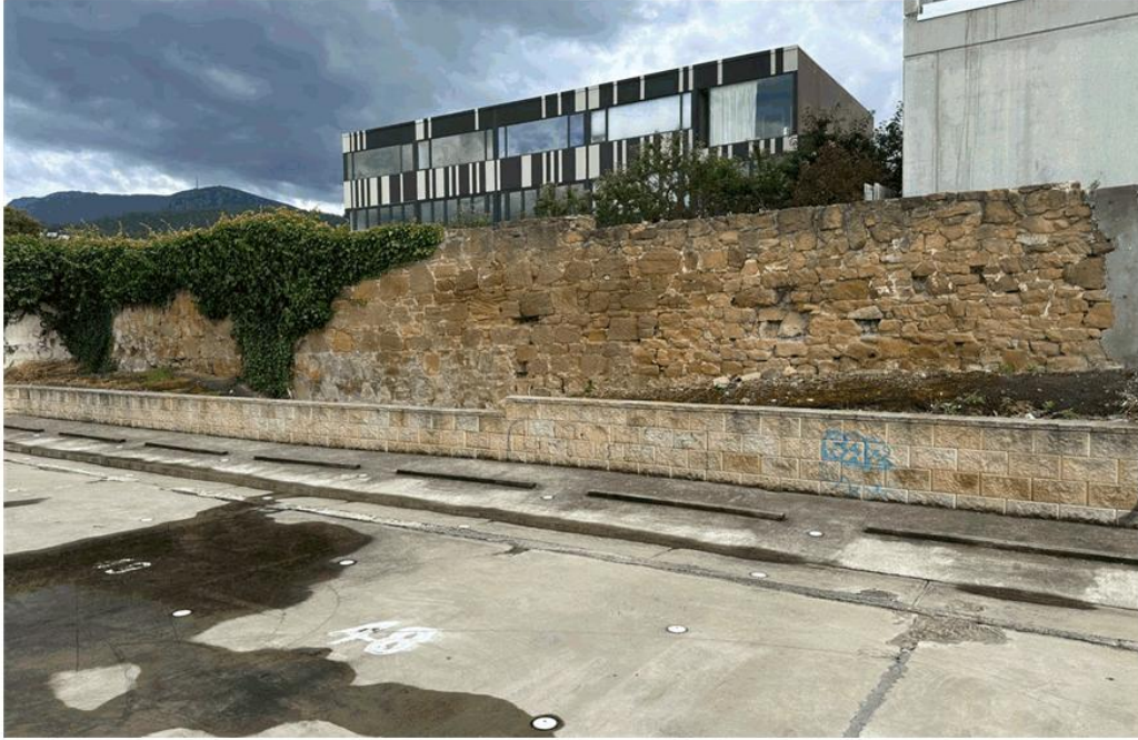
Figure 7.5 – Retaining wall at the base of the historic stone wall, indicating excavation in front of that wall.
