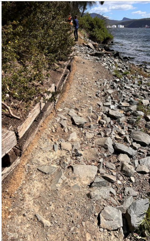
Figure 2 – Section of eroded track at waters edge on RTBG land
