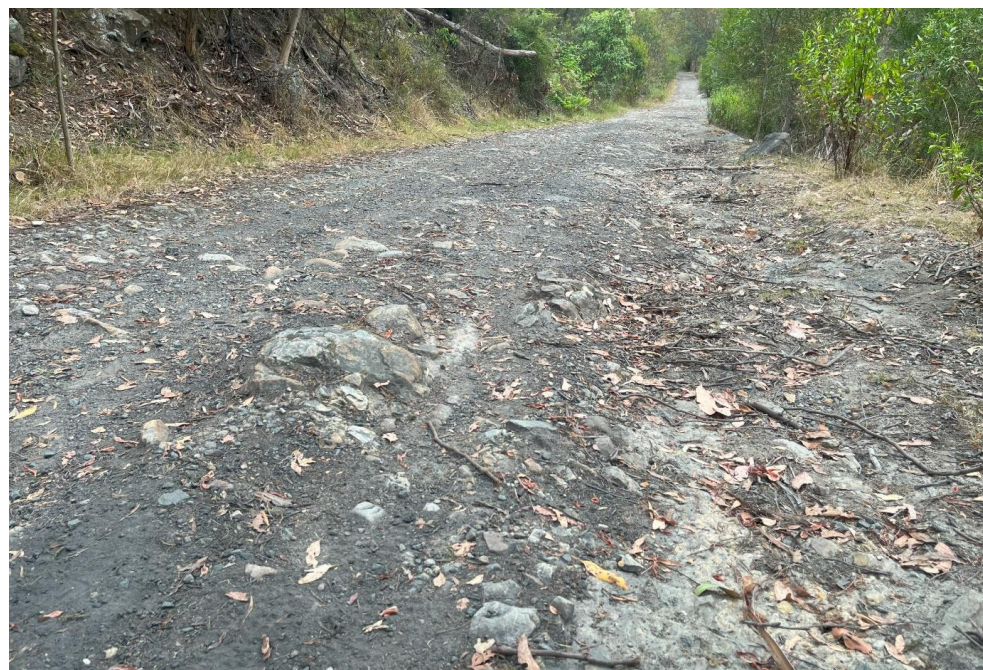
Condition of Marlyn Road Fire Trail – January 2024
