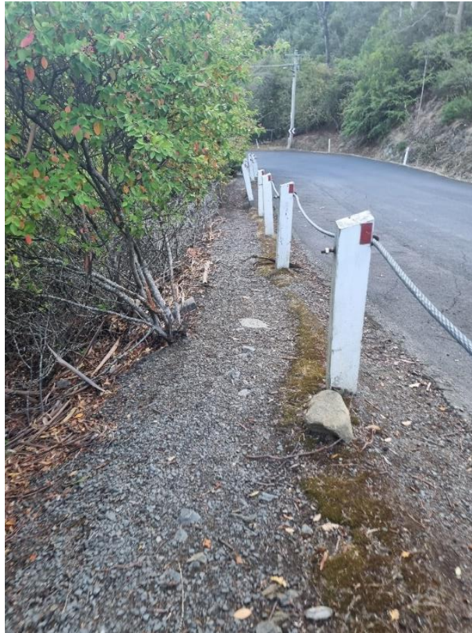
Photo 1 - Steep embankment on Rivulet bank edge on Romilly Street looking southwest towards Bridge
