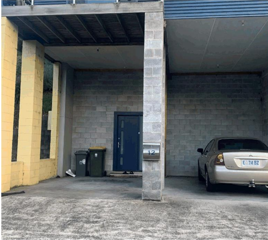
Fig. 5 - existing double carport below the multiple dwelling. Both car parking spaces will be dedicated to the proposed use
