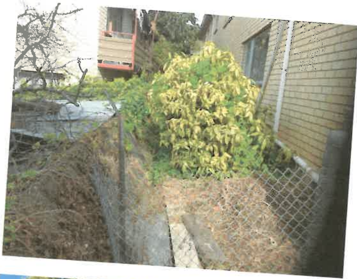
Inaccessible access to downstairs flat due to collapsing retaining wall
