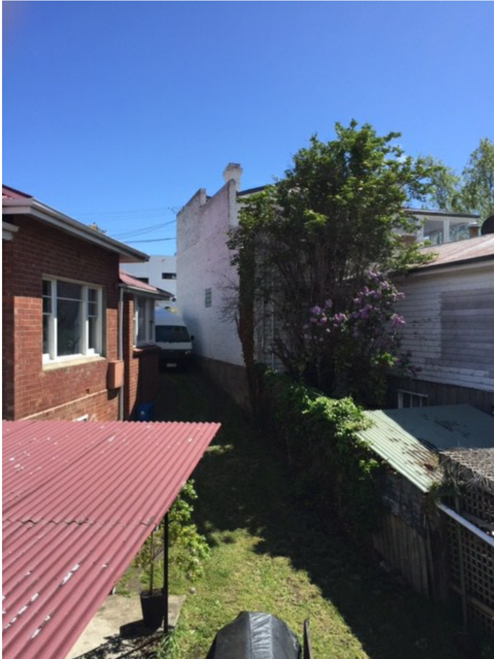
Figure 3: Looking from the deck (to be demolished) back up the driveway, noting the narrow access.
